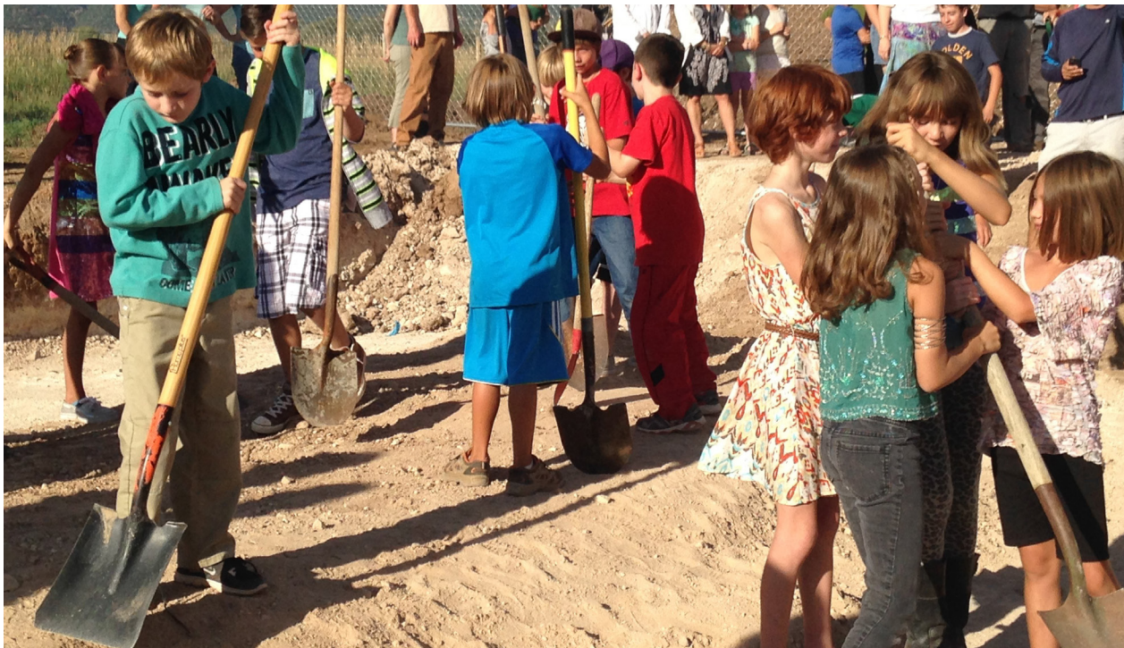
Students from Anansi Charter School in Arroyo Seco, NM help with the ground breaking to begin expansion of their new school.
