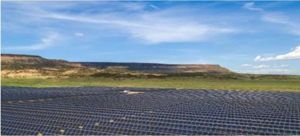
Route 66 Solar Energy Center in Cibola County
