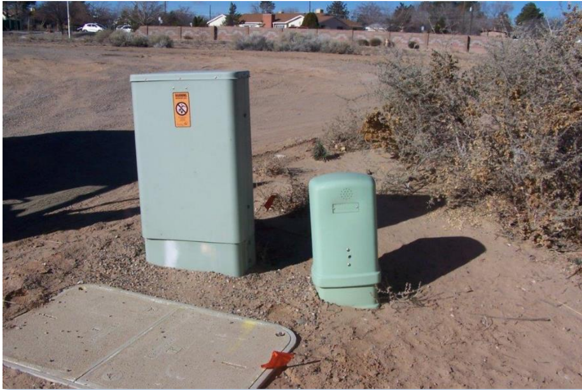
Figure 48: Rio Rancho Buried Telephone Infrastructure
