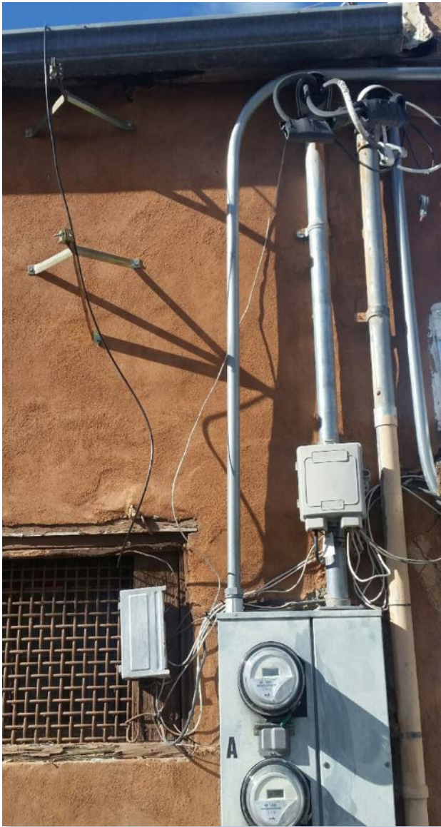
Figure 39: Downtown Santa Fe – Assorted Cables to Rooftop
