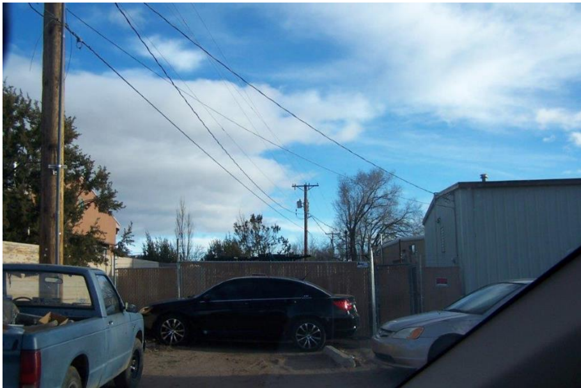
Figure 47: Rio Rancho Copper Telephone Lines
