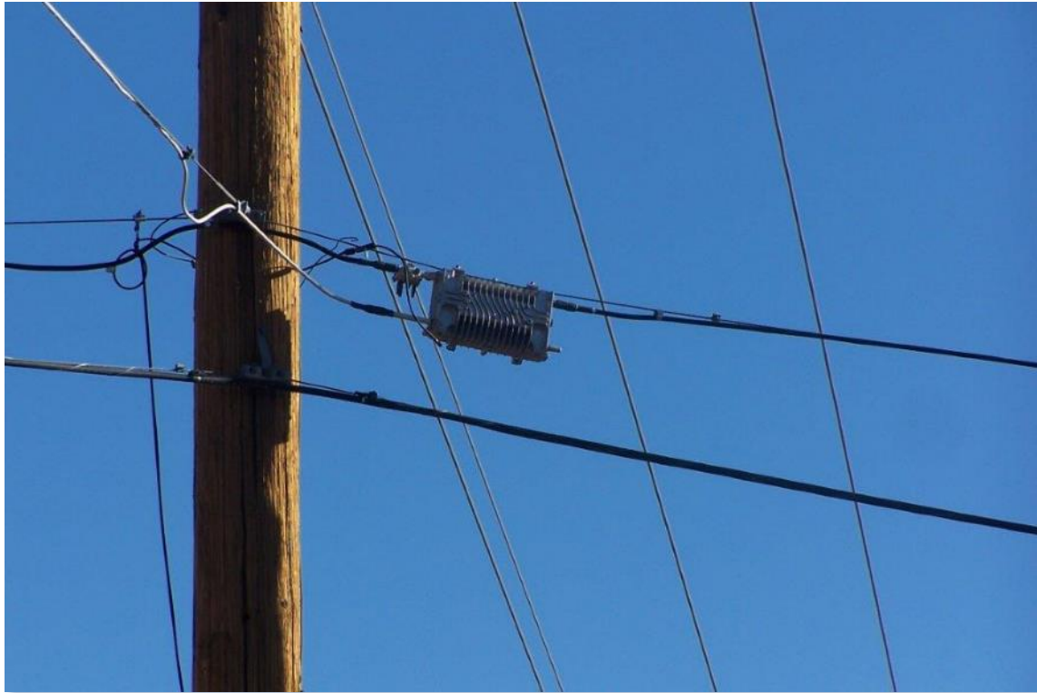
Figure 49: Reservation Area CATV Infrastructure
