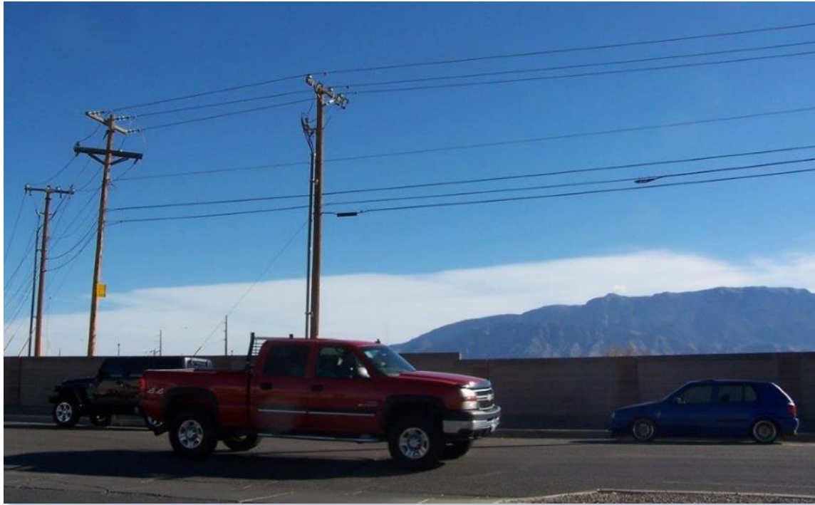
Figure 46: Rio Rancho Copper Telephone Lines
