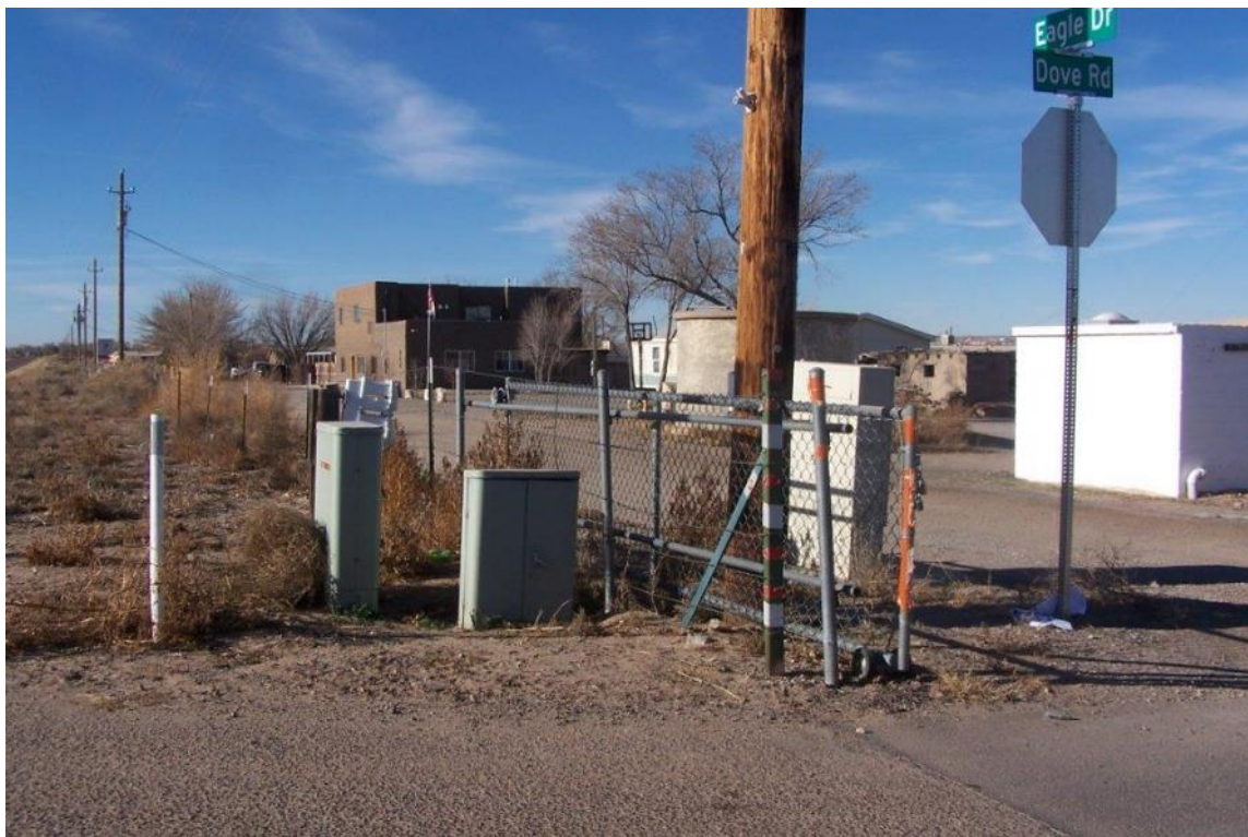
Figure 50: Reservation Area Copper Telephone Infrastructure
