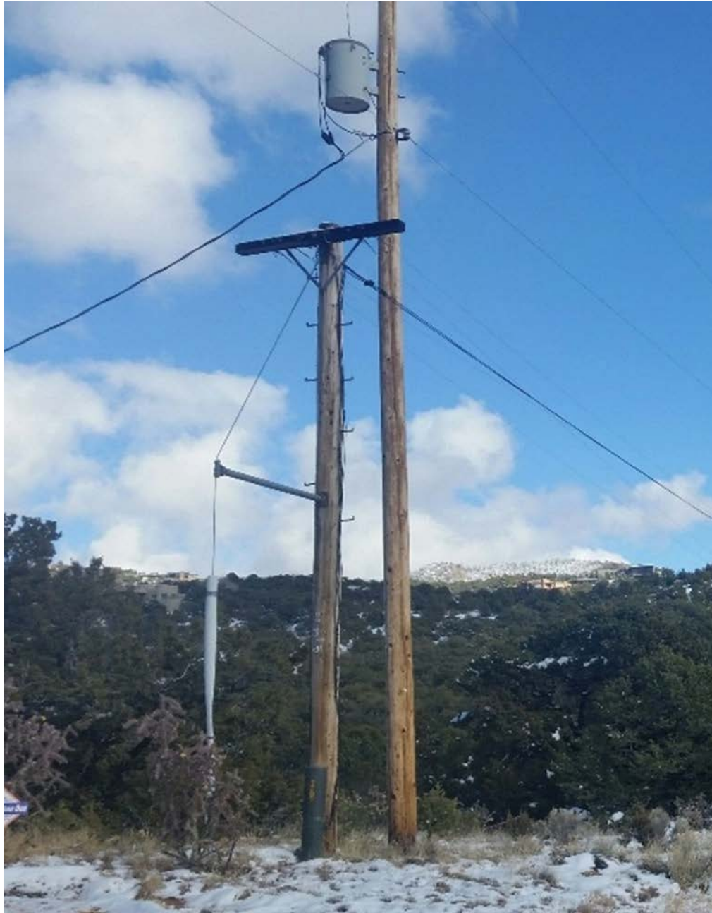
Figure 44: Old Santa Fe Trail – Poles with Ample Space for Broadband Attachment
