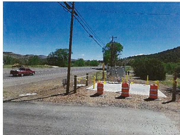
Ruidoso Downs Wastewater Collection System New Lift Station on Highway 70 Funded by CO SAP and CIF
