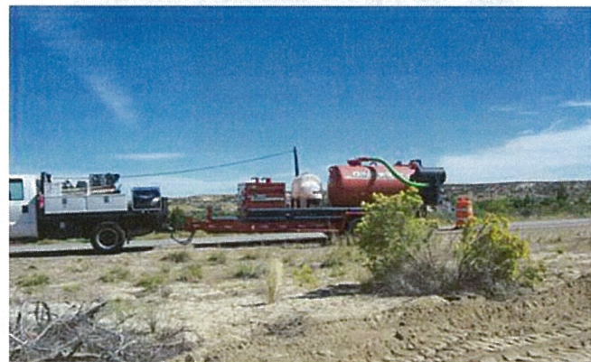
Upper La Plata MDWC Equipment to Excavate Around Existing Gas Lines For Water Capacity Project Funded by CO SAP and NMFA-DW
