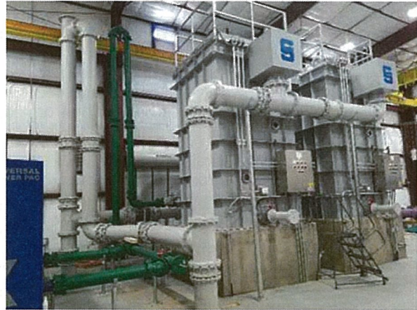
Clovis Reuse System Phase 1B, Additional blower Filter Unit Funded by CO SAP and WTB
