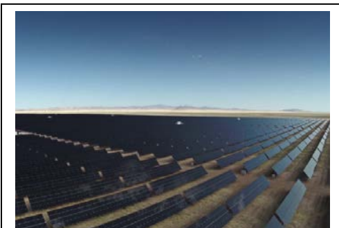
An existing solar facility: Macho Springs Solar in Luna County. Photo courtesy of Solar Builder Magazine.
