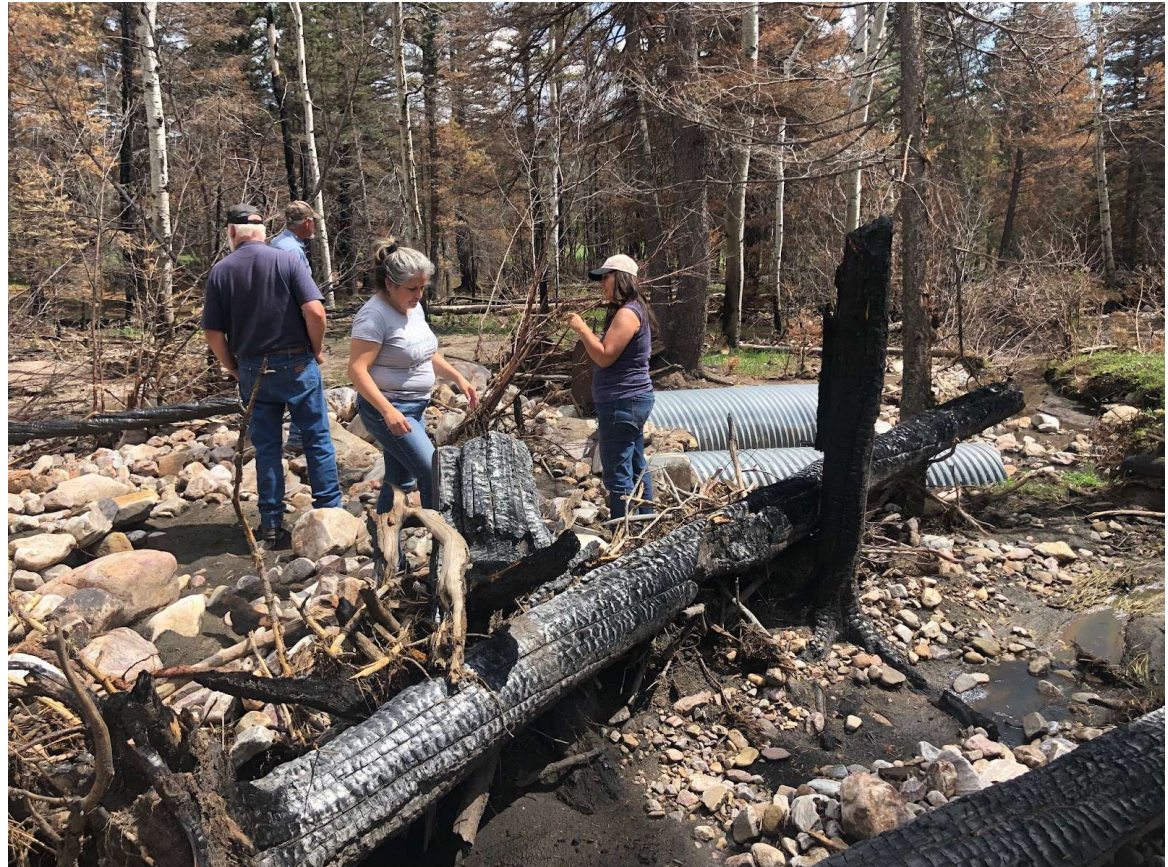
Heavy debris flows destroyed the diversion for Acequia del Sombrillo in Mora County after the HPCC fire and post-fire floods. This area is prone to recurring flooding (cascading events).
