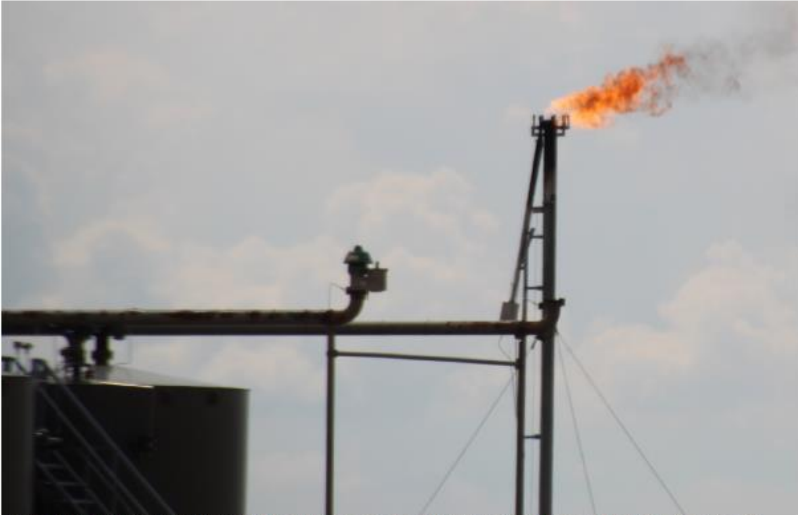
A poorly lit flare at Rustler Breaks SWD #6/ API #30-015-45034, a San Mateo Midstream facility in Eddy County, New Mexico, Sept. 2022. Photo credit Charlie Barrett, Earthworks.
