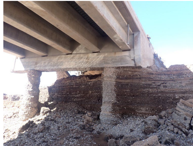
Bridge 9030 (US-285 SB @ MP 88, south of Roswell, north embankment was washed out by large flood.
