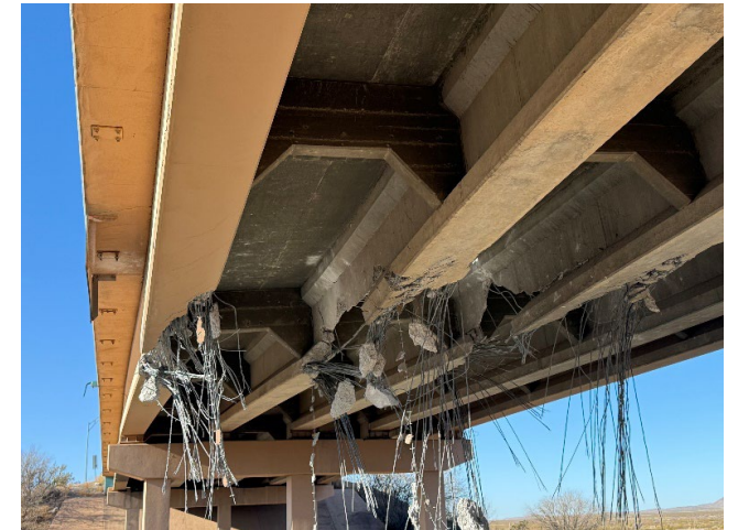
Bridge 7301 (Lordsburg interchange bridge, I-10 WB @ exit 24) was struck by an overweight vehicle.
