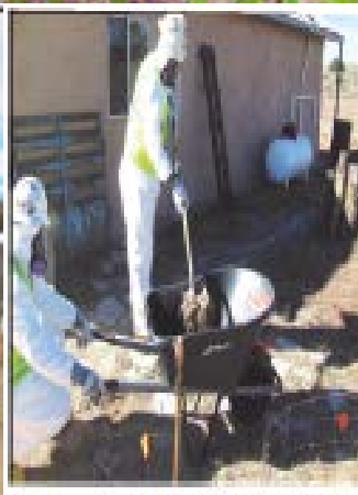
Hogan Mine Area—contaminated parking rocks at residence were removed
