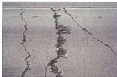
Spalling of transverse cracks
