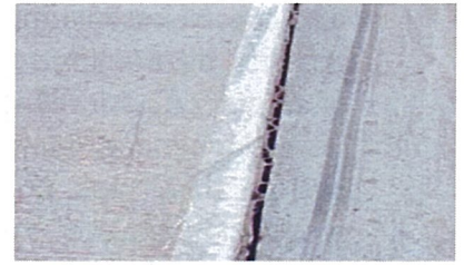
Joint Seal Damage
