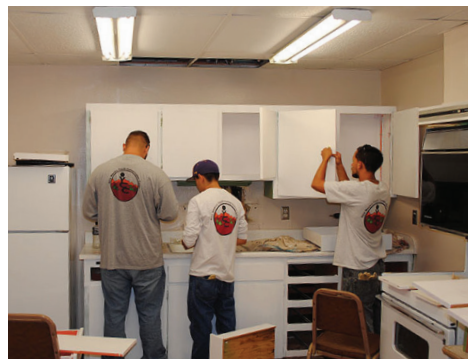
Teaching Trades Corps members remodel the kitchen at the Del Norte Community Center Enhancement Project. Project Sponsor-City of Tucumcari, Quay County
