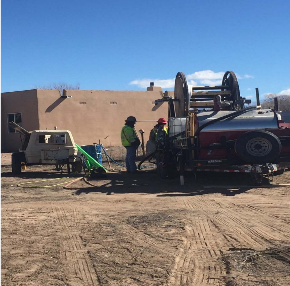
San Ildefonso Pueblo Waste Water System
