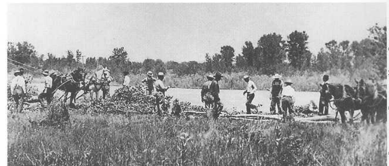
W. R. GIBSON PHOTO CAPTURES CREW PERFORMING RIPRAP WORK ON THE ANIMAS RIVER TO DIVERT WATER INTO AN IRRIGATION DITCH.
