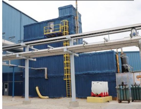
Molten Salt Purification Plant Elmore, OH
