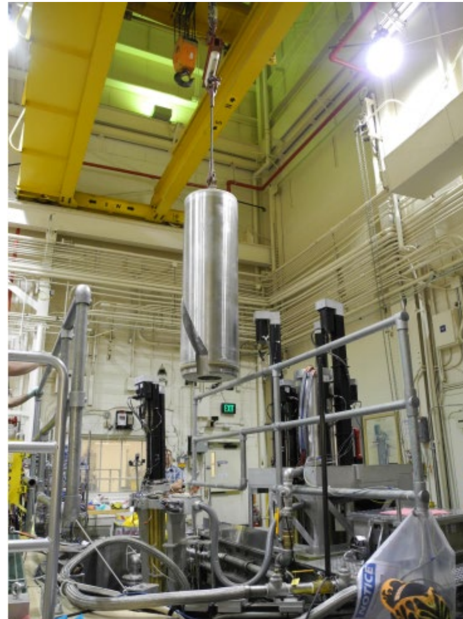
Current overhead crane in the Annular Core Research Reactor high bay.
