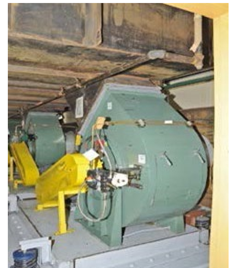
Ventilation system fan planned for replacement.
