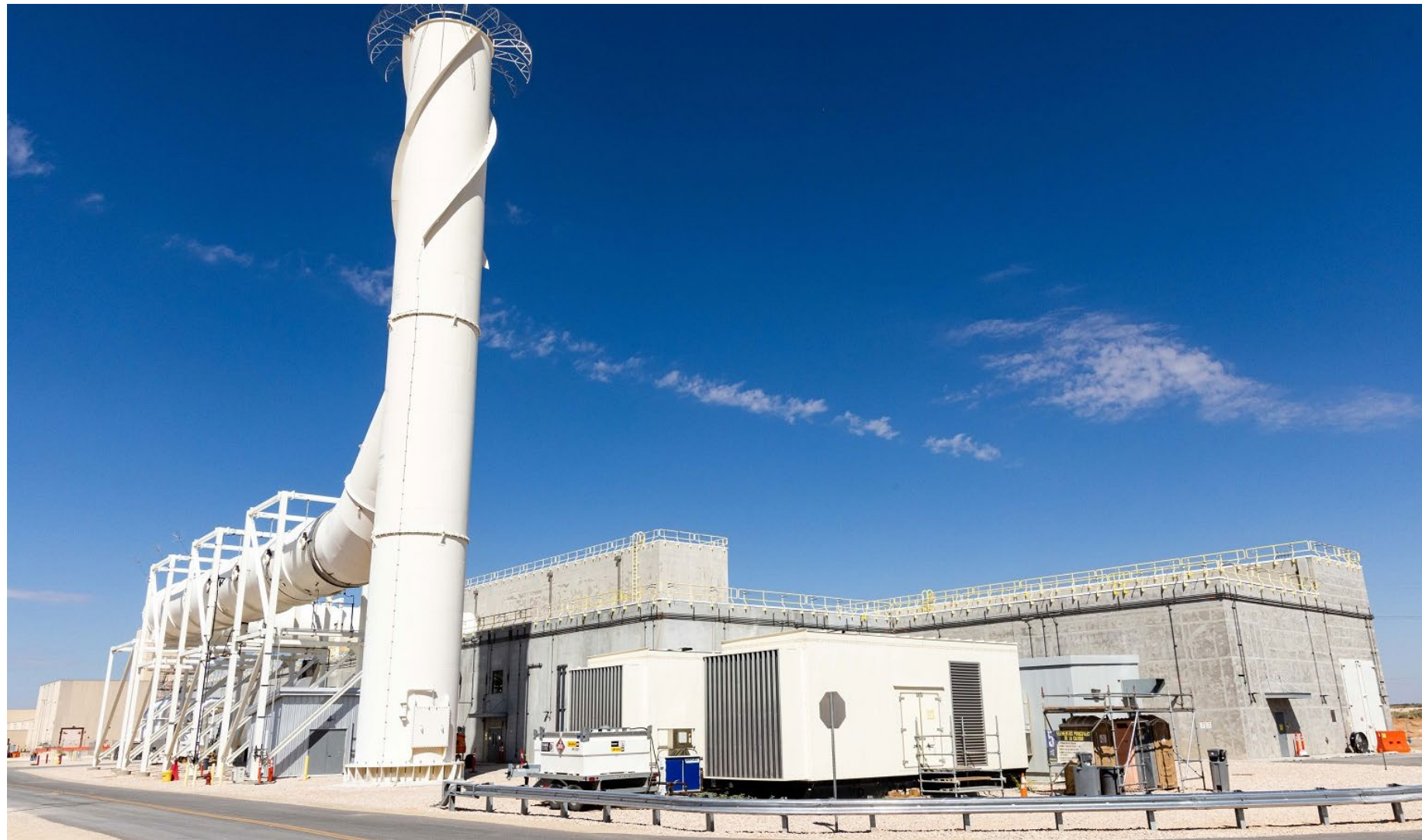
Underground Ventilation System
