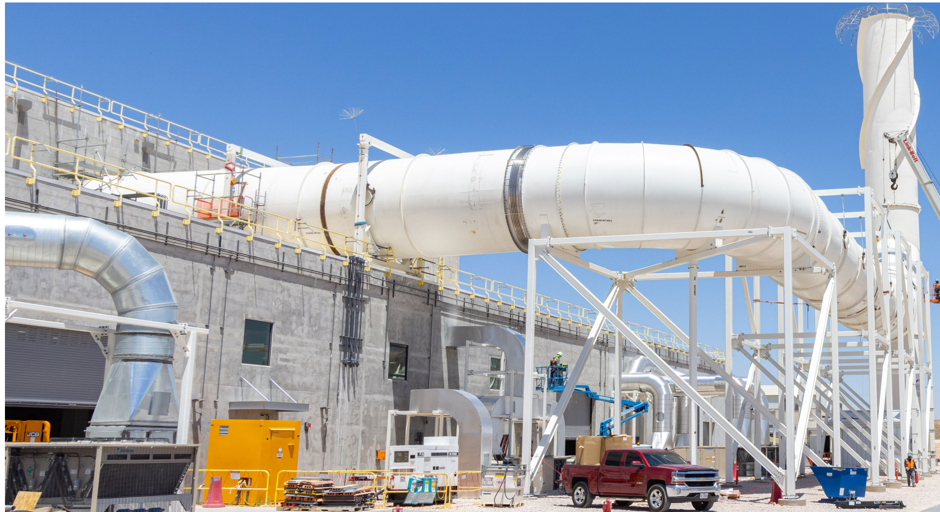
UVS, formerly known as the Safety Significant Confinement Ventilation System
