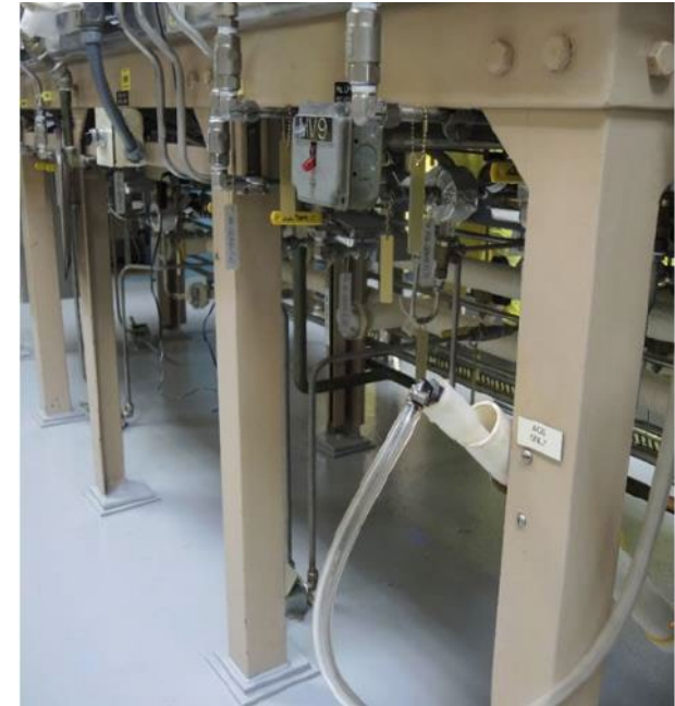
Seismically Deficient Glovebox Stand
