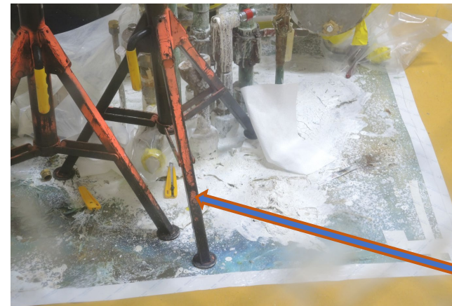
Unsecured sharps in high contamination area
