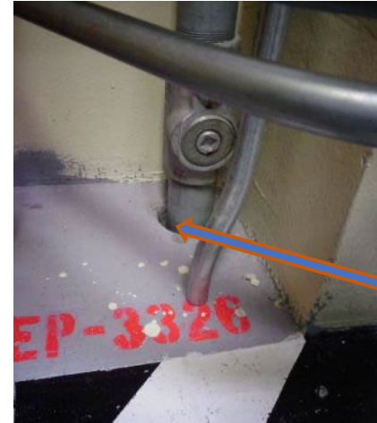
Unsealed fire penetration in PF-4
