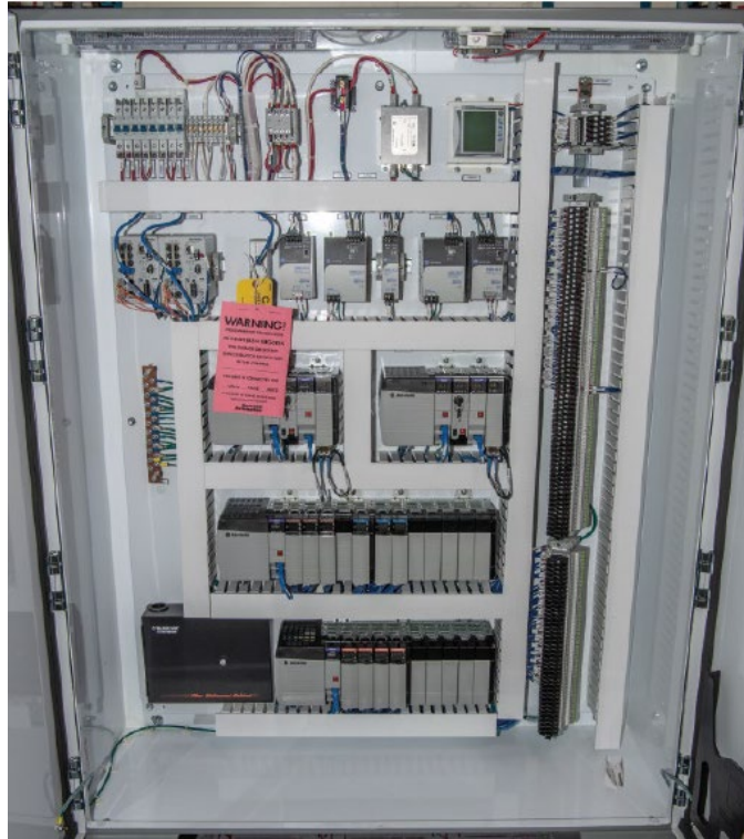
New Facility Control System Components
