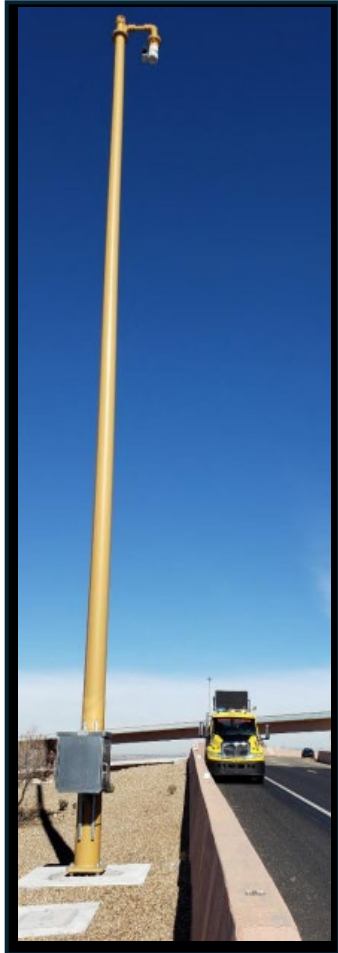
Closed Circuit Television Systems
