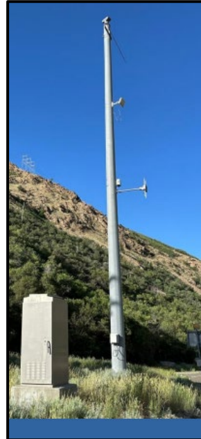
Traffic Sensor Systems
