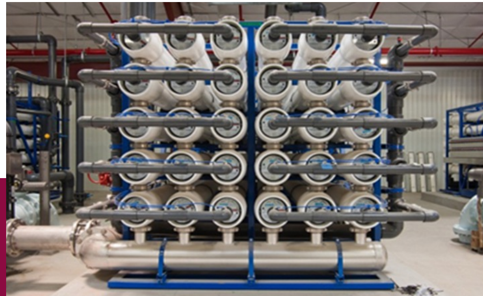
Typical RO Skid (1 MGD Unit)
