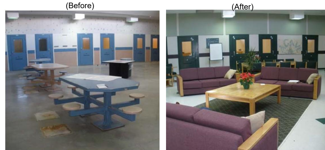
Remodeling at John Paul Taylor Center CYFD Juvenile Secure Facility in Response to New Mexico’s “Cambiar” Initiative
