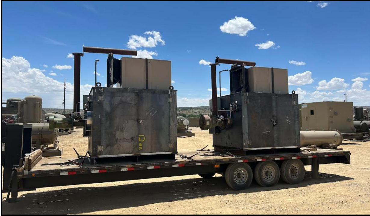
Navajo Tech-NMT-Navajo Nation Water Purification Project – Working to Desalinate brackish water wells on the Navajo Nation
