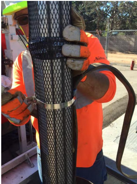
Sacrificial anode added to extraction wells to prevent corrosion
