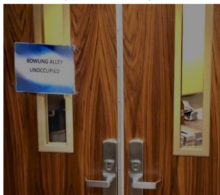
Figure 3. Unfinished Bowling Alley at NMVH Annex
