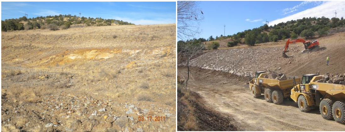
Photo on the left shows the lower portion of the tailings impoundments where tailings (yellow material) had been exposed by erosion. Photo on the right shows the same area after the placement of cover material, re-grading, and armoring.
