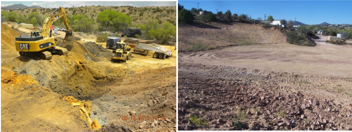
Photo on the left shows the removal of tailings. Photo on the right shows the same area after the tailings and contaminated soils were removed followed by the placement of clean backfill, re-grading, and re-seeding.
