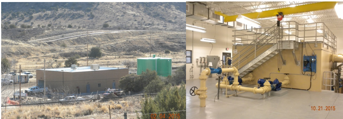
Completed construction of the wastewater building and the 20,000-gallon above ground storage tank. Photo on the right shows equipment installed in the new building.
