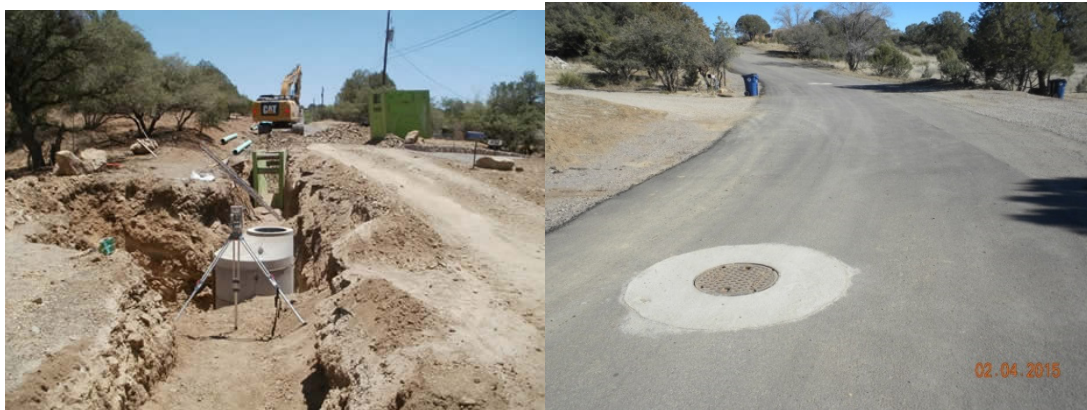
Photo on the left shows trenching for sewer line and manhole installation. Photo on the right shows the area after the sewer line was installed and the trench had been backfilled, compacted, and asphalted.
