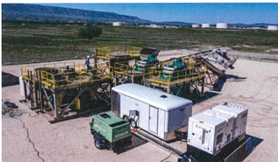
A commercial HPSA™ circuit like the one that will be used.
