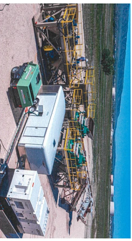
10 TPH HPSA™ circuit setup
