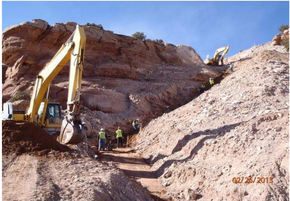
Backfill utilizing bedding material around the HDPE pipe. 12" HDPE WL down the Slope of the Mesa Cliff Worksite WS-21A.
