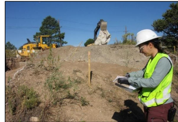
As part of the Southern External Boundary Campaign, a geologist assesses excavation of contaminated soil in Lower Water Canyon
