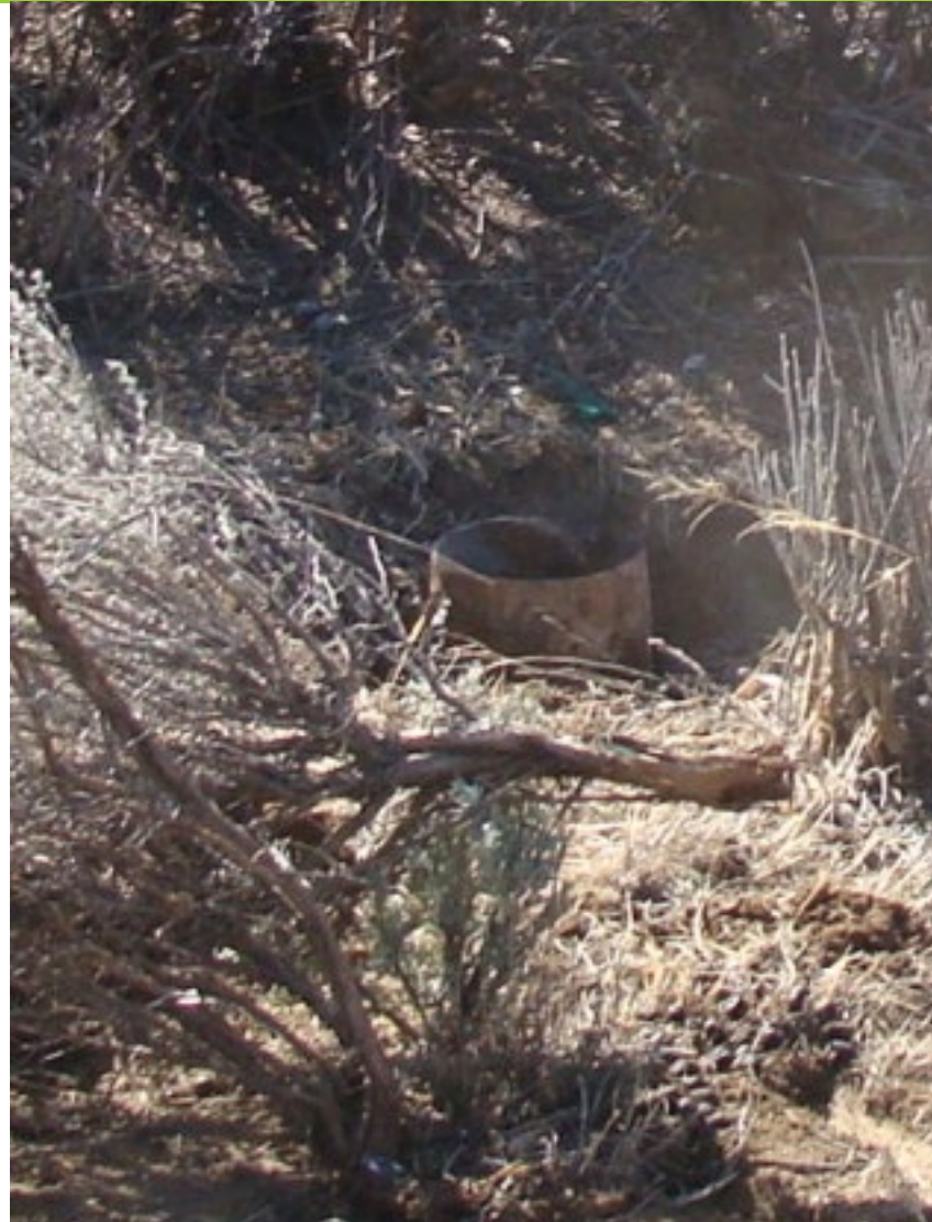
Abandoned Well previously buried underground
