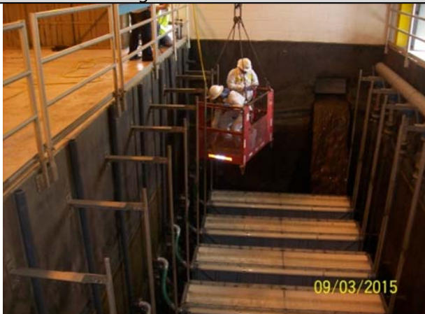
Los Lunas Existing and New MBR Cassettes Installed
