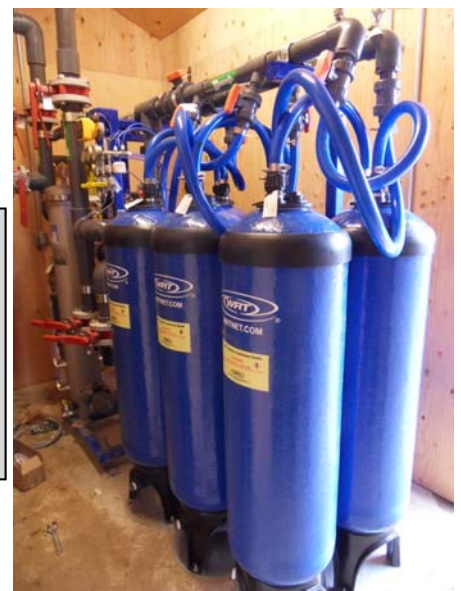
Upper Arroyo Hondo Uranium Treatment System
