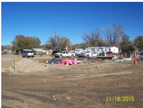
San Juan County Lower Valley Lift Station Site Funded by CWSRF
