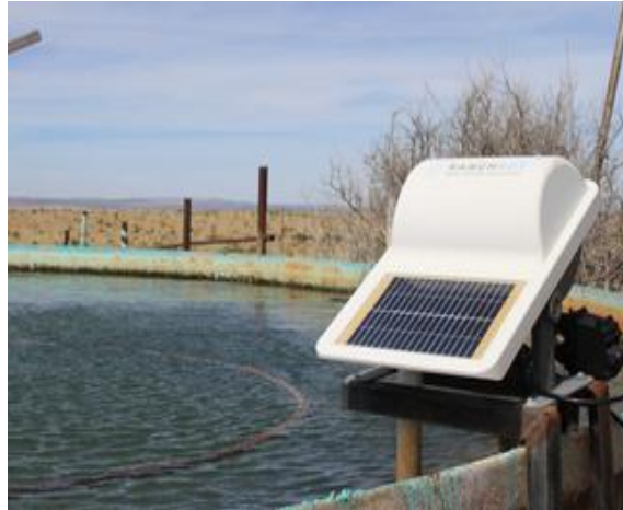
Water Tank Level Monitor
